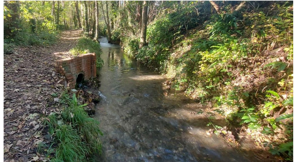
Run off from the road network entering the stream through a brick outfall
